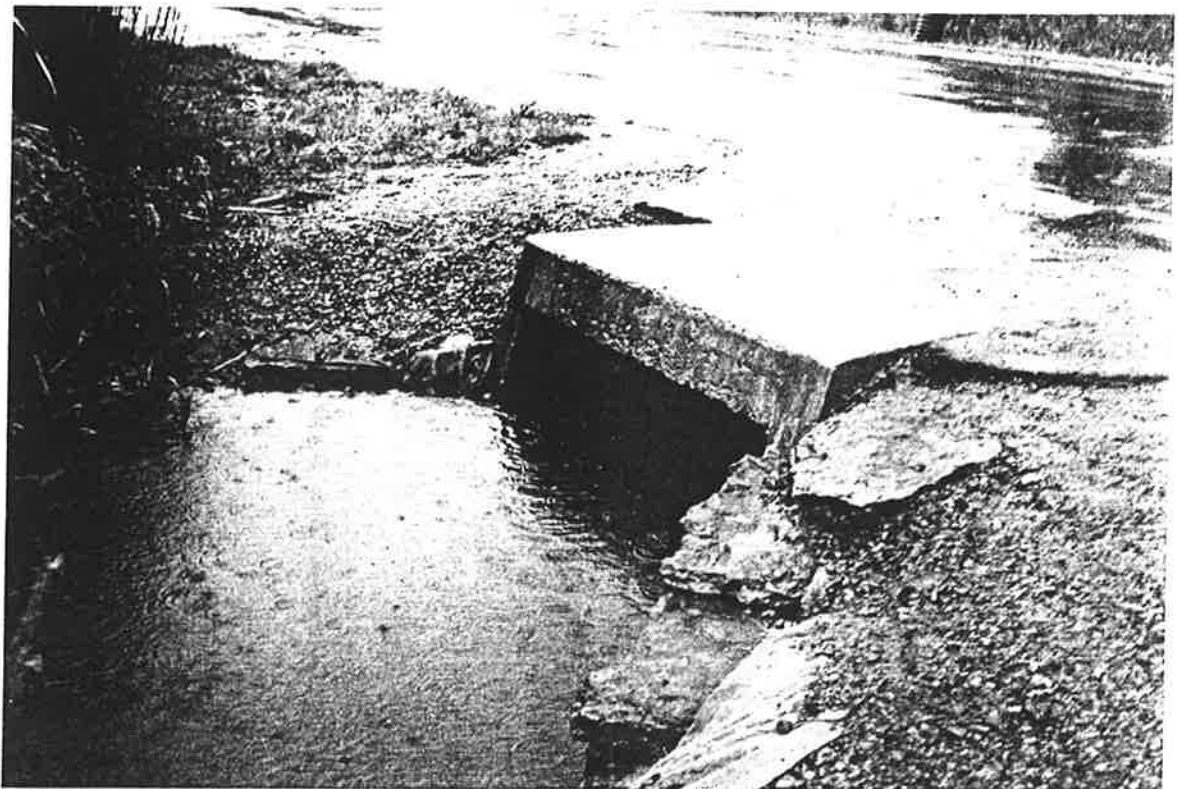
#4 - AT POINT B ON EAST SIDE
